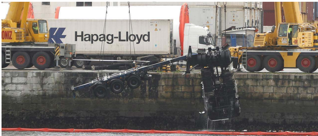
This was the retrieval of the truck that fell to the Guixar FDV PIER
